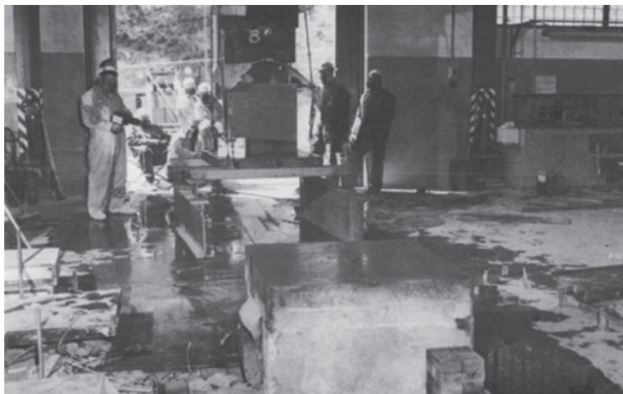
Figure 6. Removing the remainder of the tamper required the welding of two 4" I-beams to the supporting plate below the tamper unit. The beams were welded onto skids made of larger I-beams so the assembly could slide across the floor and onto the adjacent loading dock, where it was loaded onto a truck for transportation to the South Mesa contaminated area and covered with a wooden shack for protection against the weather.
